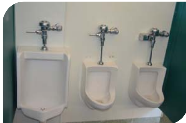
Restrooms need to be modernized.
