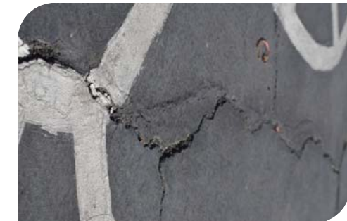
Blacktop and parking areas must be repaired.
