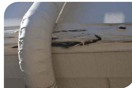
Deteriorating surfaces should be repaired.
