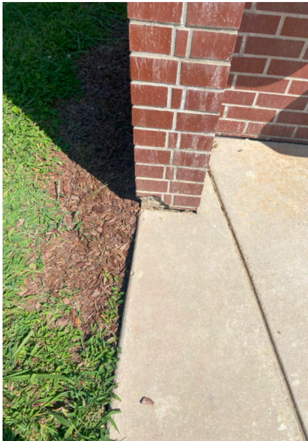
Damage to exterior brick
