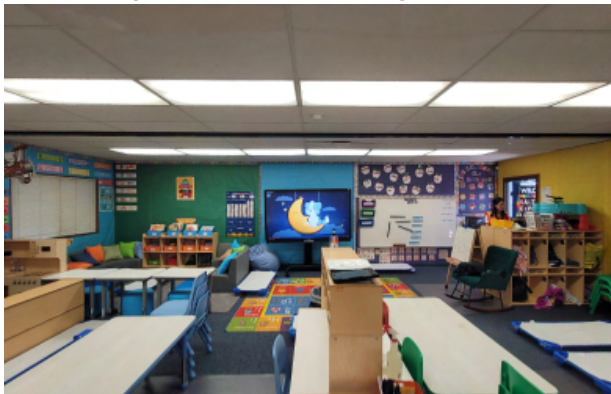
Ceilings showing signs of damage
