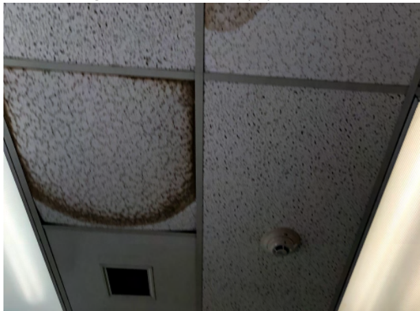
Major water damage to ceiling tiles
