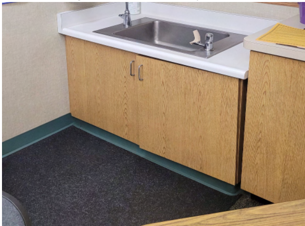
Casework is damaged in classrooms
