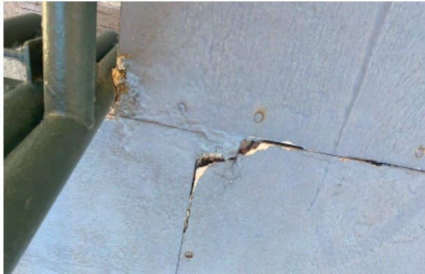
Cracks/damage to wheelchair ramps
