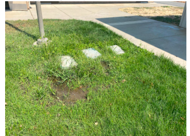
Water overflowing on lawn from plumbing
