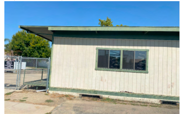
Portable exterior damage
