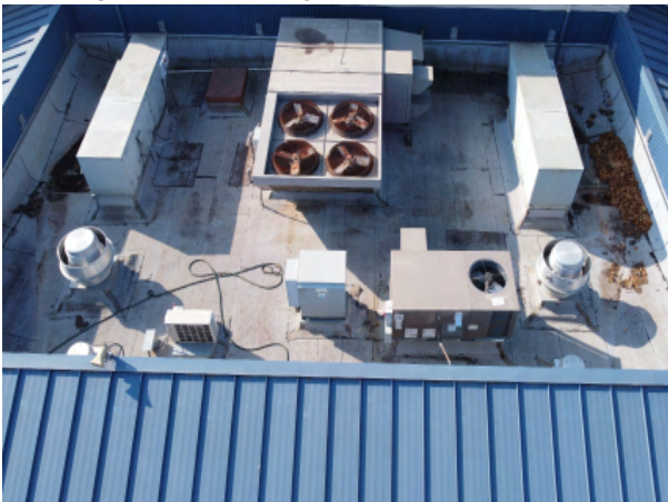
Mechanical equipment and roof aging
