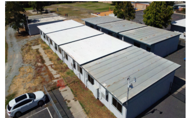
Portables in major need of repair
