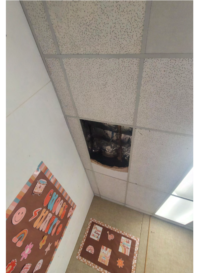
Missing or damaged ceiling tile
