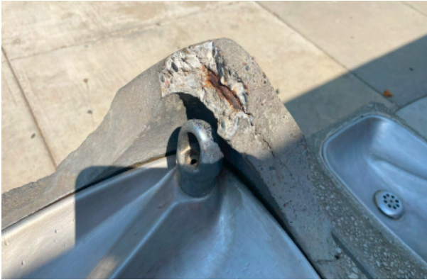
Drinking fountain damaged/broken
