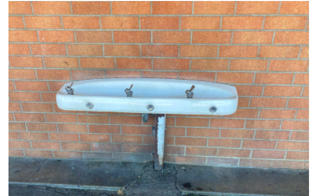
Drinking fountain area damaged
