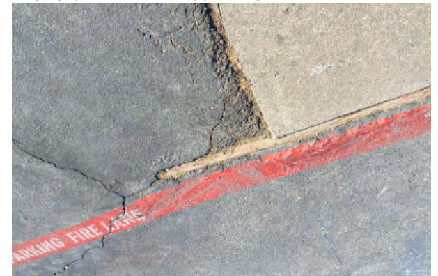
large gaps and cracks appearing on concrete
