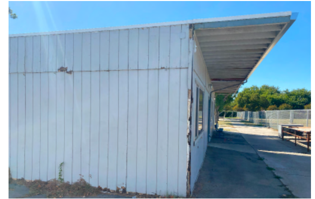
Portables in major need of repair
