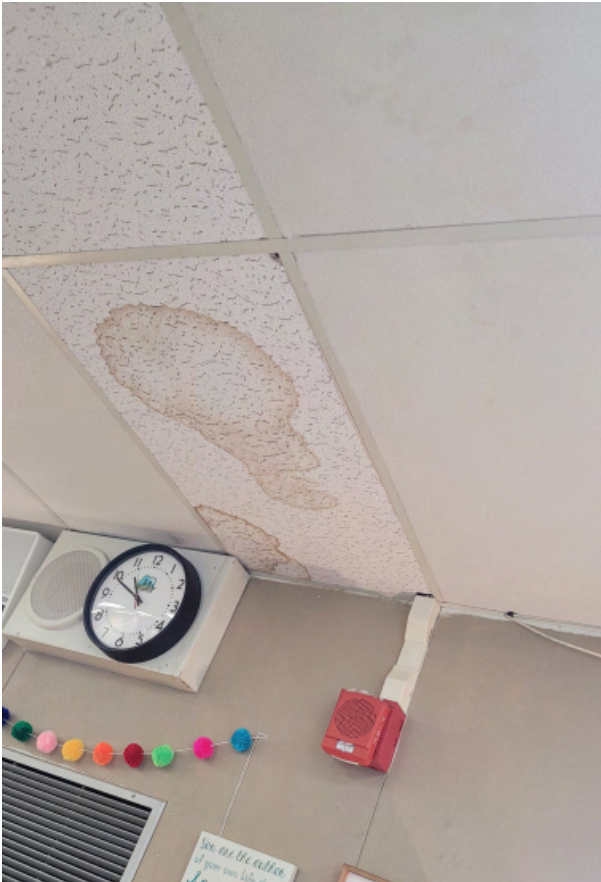
water damage on ceiling tiles
