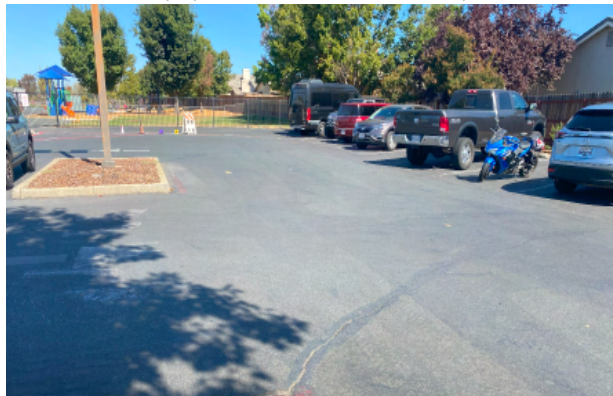
cracks appearing on asphalt
