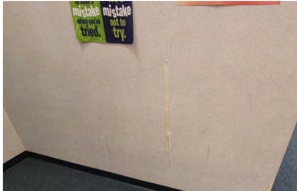
walls have wear and tear
