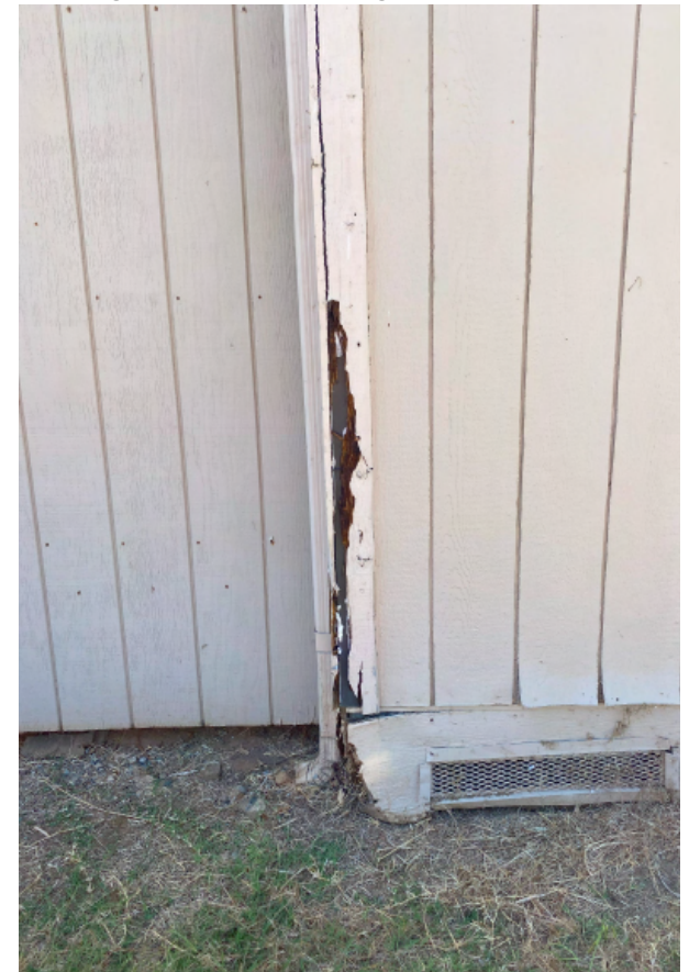
Exterior wall breaking away
