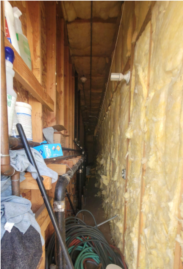
Exposed insulation and safety hazards
