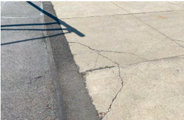
Cracks appearing on blacktop
