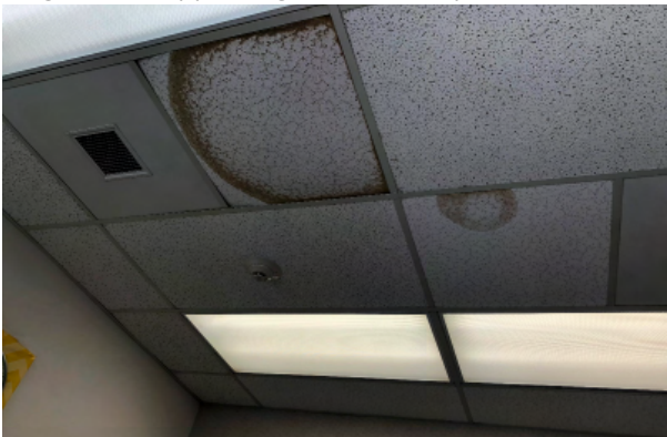
Water damage on ceiling tiles
