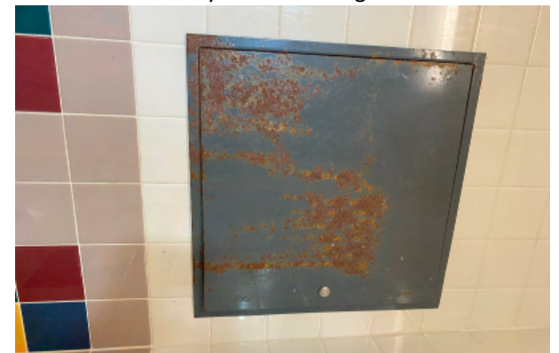
Rust and age affecting restroom equipment
