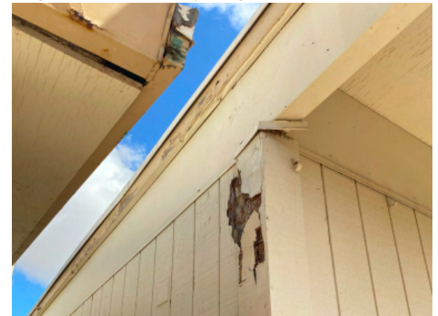
Exterior walls show signs of age and wear
