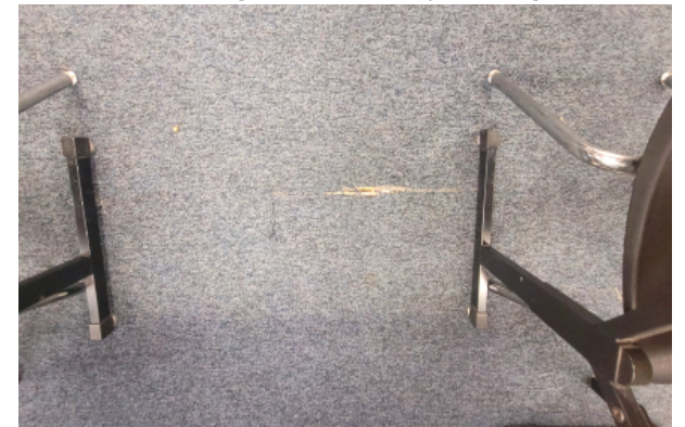
Carpet in classroom has tears
