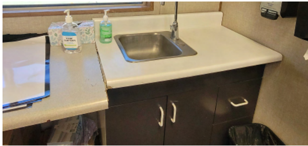
Casework showing signs of damage
