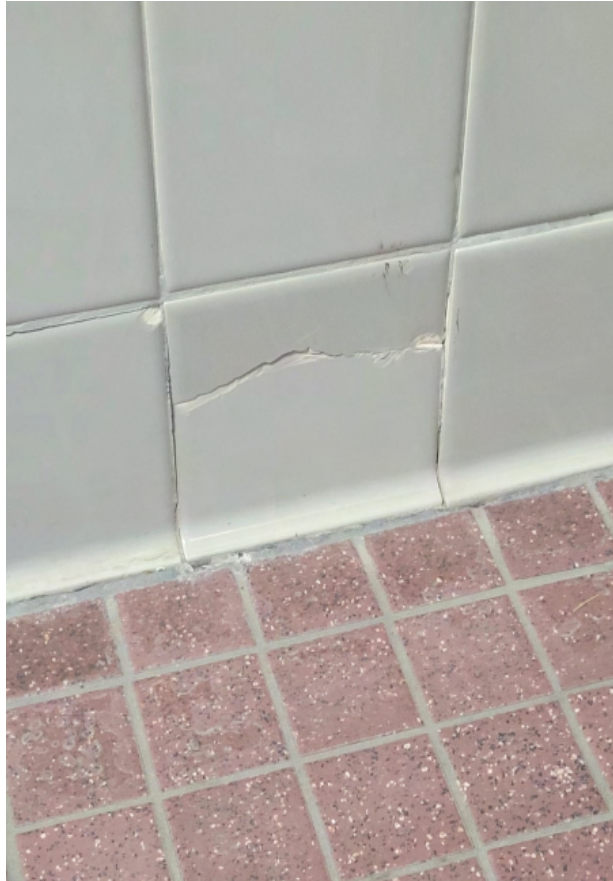
Restroom tiles are cracking
