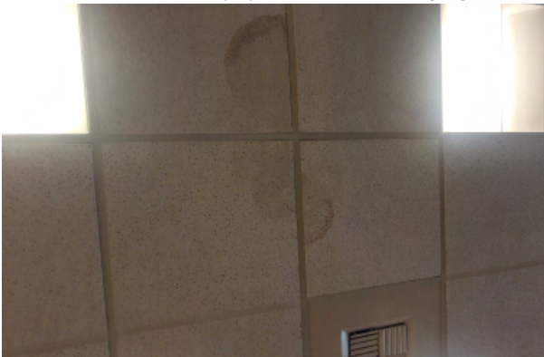
Water damage to ceiling tiles
