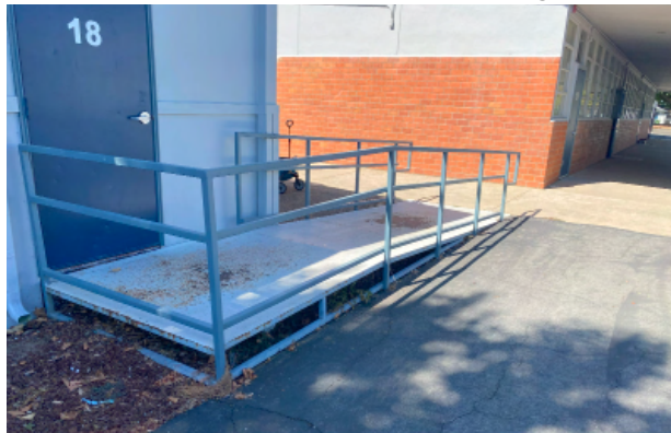
Ramps have sign of wear and tear
