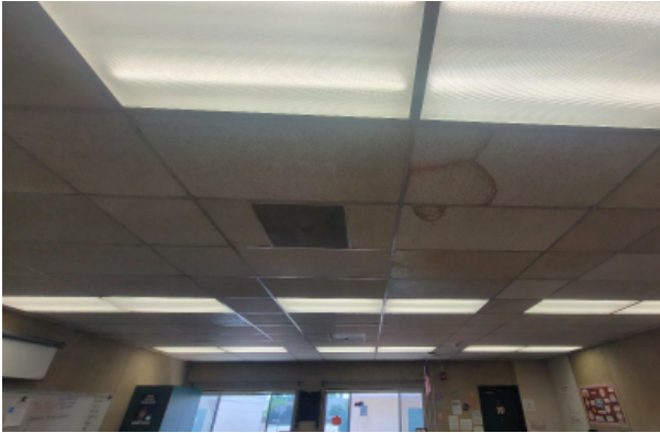
Water damage has affected the ceiling tiles
