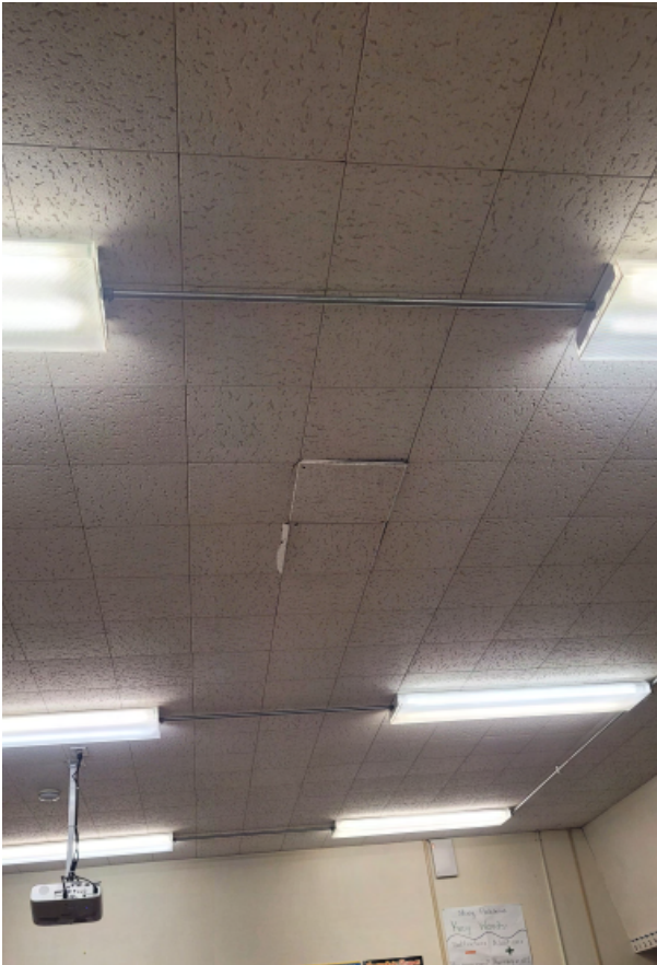
Damage to ceiling tiles
