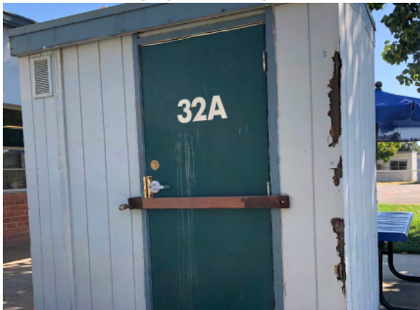
Small storage closet exterior damage
