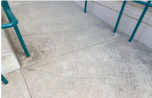
Cracks appearing on ramp walkways
