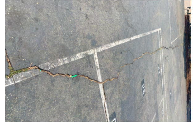
Cracks appearing on asphalt
