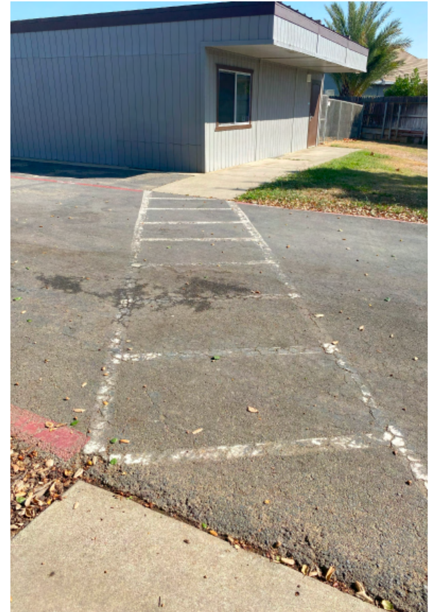
Gaps between asphalt and concrete
