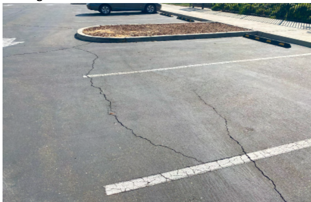
Cracks appearing on parking lot asphalt
