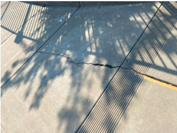
Large cracks appearing on concrete paths
