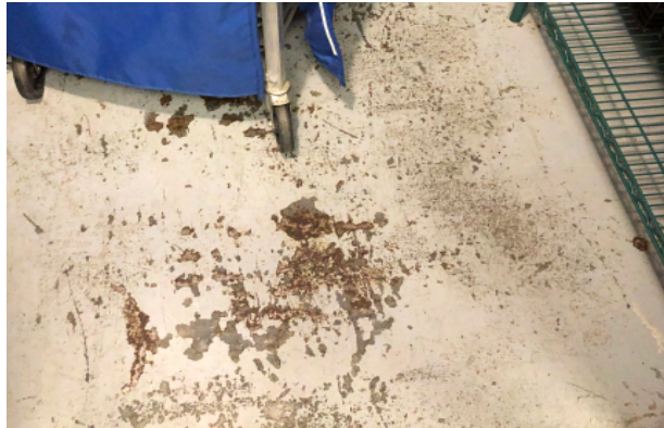
Floor damage due to kitchen equipment
