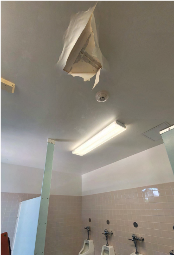
Large tear in ceiling finish
