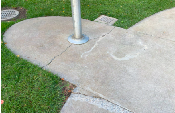
Cracks appearing on concrete
