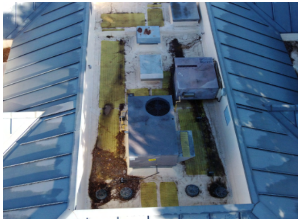
mechanical equipment and roof are dirty
