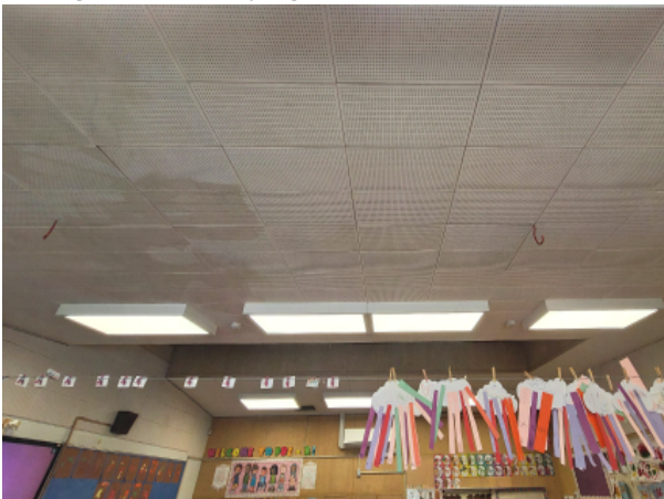
Water damage to ceiling tiles
