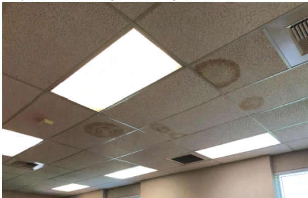
Water damage to ceiling tiles
