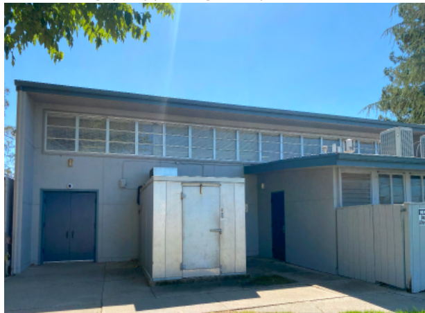
Concrete cracked and wooden fence damaged
