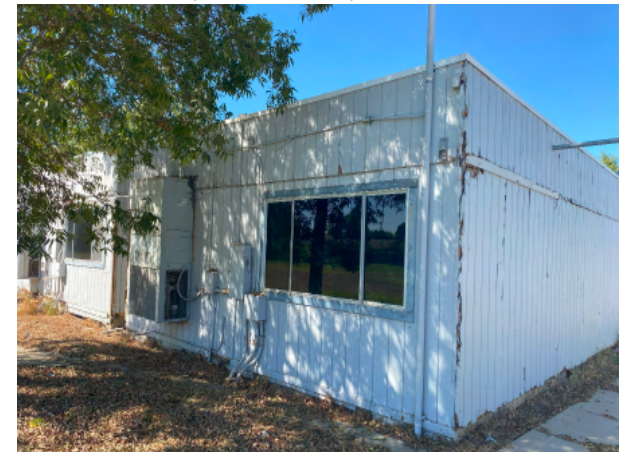
Portables in major need of repair
