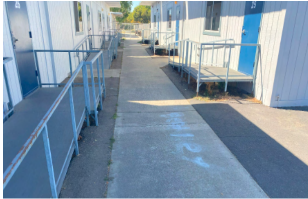
Cracks and gaps appearing on asphalt
