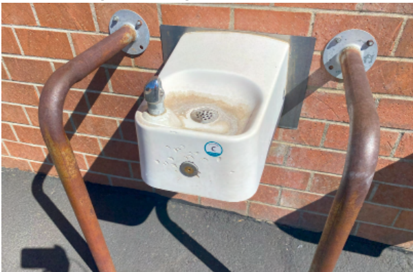
Drinking fountain damaged
