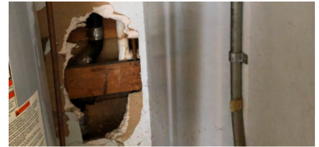
Large holes on walls exposing internals
