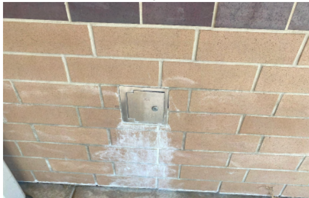
Water dripping on exterior wall leaving deposits
