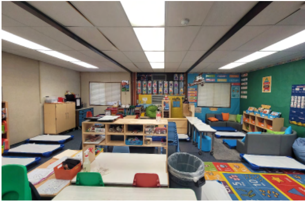
Ceiling tiles are warping
