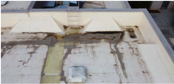
Roofs aging and dirty
