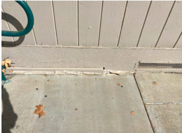
Poor quality of construction/maintenance
