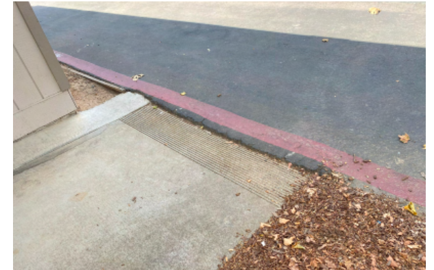
Large gaps/cracks appearing on asphalt
